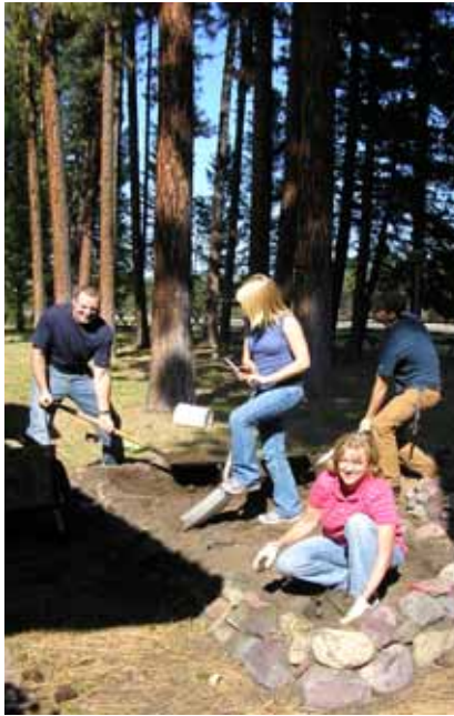
Seeley Swan High School students and staff helping to construct pollinator garden beds.
